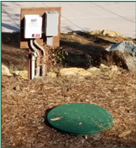
Typical STEP system control panel and lid
