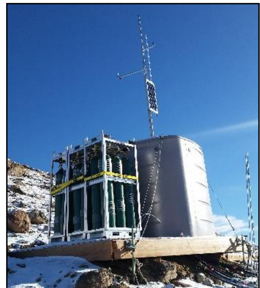
Typical Gazex Shelter
